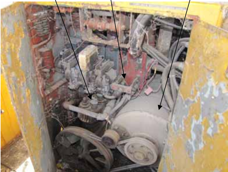
COMPRESSOR, MAIN SWITCH & GENERATOR
