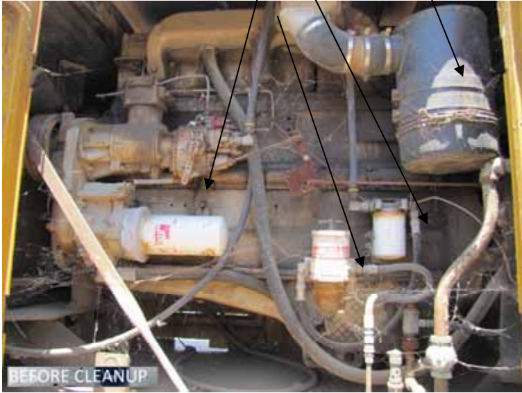
LEFT HAND SIDE FILTERS, AIR CLEANER
