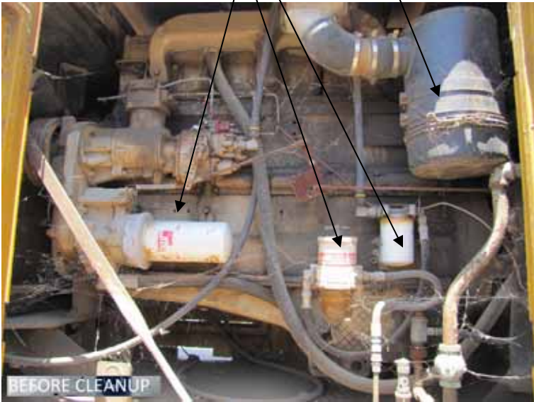
LEFT HAND SIDE FILTERS, AIR CLEANER
